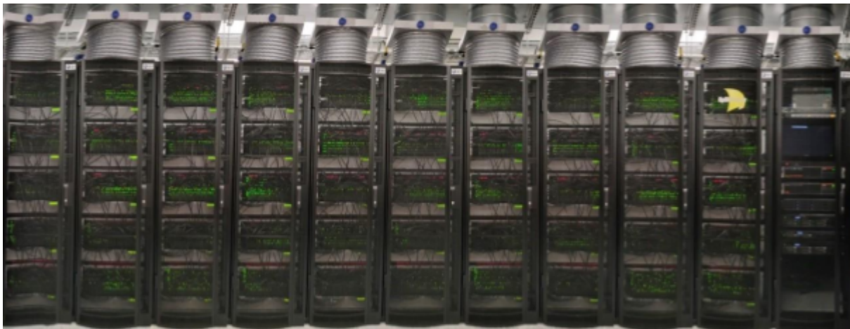
Figure 1: A 10 cabinet machine, wired together (Note: the 11th cabinet in the picture contains servers for handling jobs sent to the machine).
